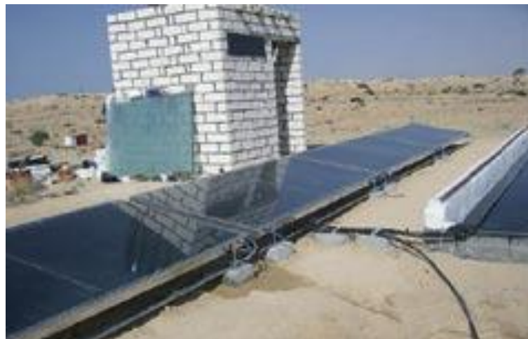
Figure 14: Small Scale Solar Unit at Omayed Biosphere
