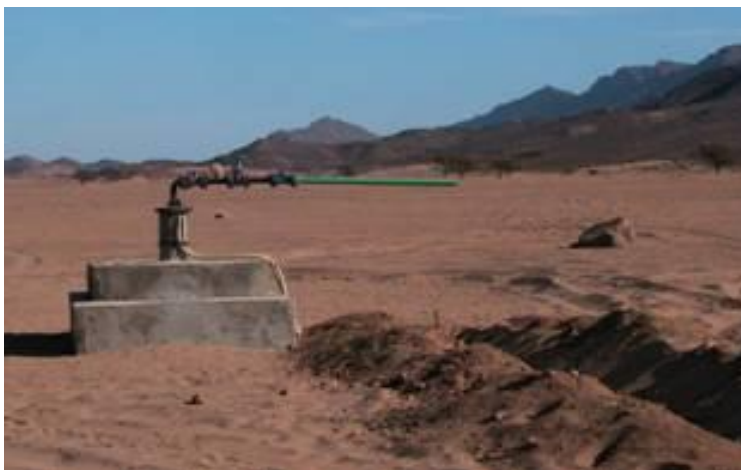
Figure 16: Controlled water extraction from a well in Abu Saafa, Elba protectorate, adjusted for drip irrigation.
